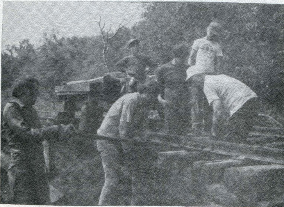
Bob Blomquist, Norm Livgard, Dave Schauer, John Vincent, Dave Fuhr, and Lloyd Berger work at site of washout near Morgan Park.
