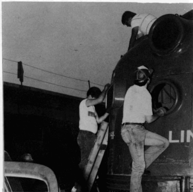
John Singer, Greg Vreeland and Tom Dorin begin restoration work on the nose of the 2500A.
