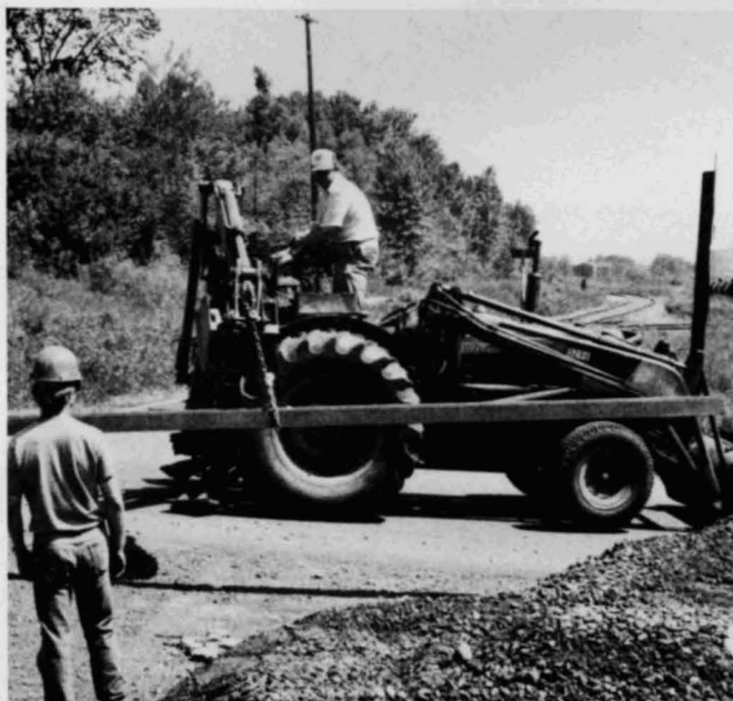
Mark Olson operates the Fordson tractor to lift rails to be moved to the Herman Avenue crossing for rail replacement.
